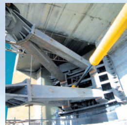
Servomotor for radial gate
